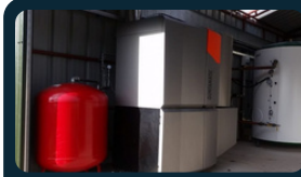
Biomass Heating and Heat Pumps
