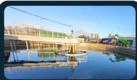
Bridge Scraper Systems
