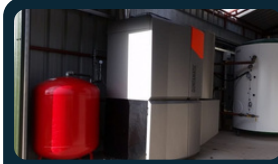
Biomass Heating and Heat Pumps
