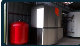
Biomass Heating and Heat Pumps
