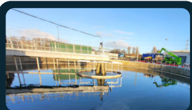
Bridge Scraper Systems
