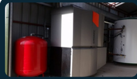
Biomass Heating and Heat Pumps
