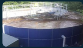
Activated Sludge Treatment
