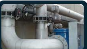
Deep Bed Sand Filters
