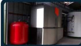
Biomass Heating and Heat Pumps
