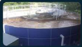
Activated Sludge Treatment
